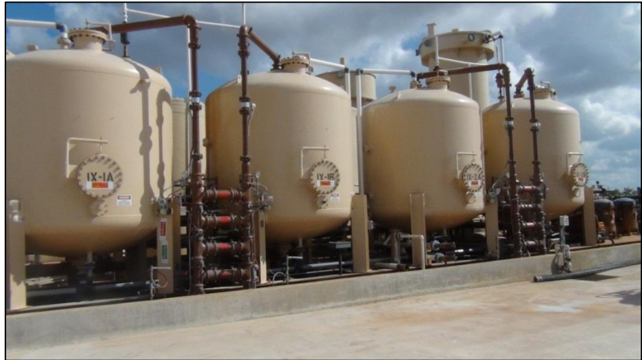
Image 1: Water processing tanks
