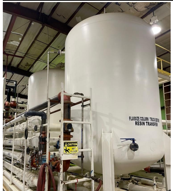
Figure 7: Inside Christensen Ranch satellite plant
