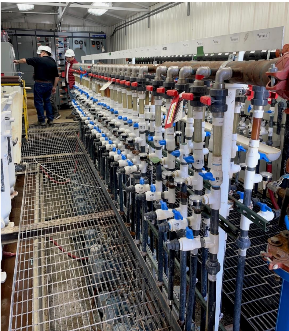
Figure 9: Christensen Ranch – Unit 8 header house
