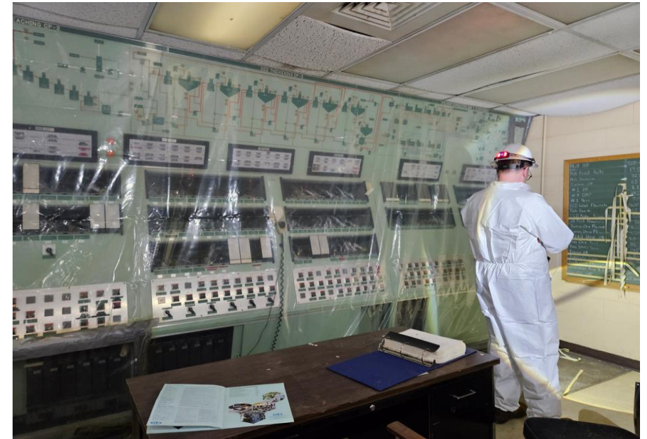
Sweetwater Plant Control Room
