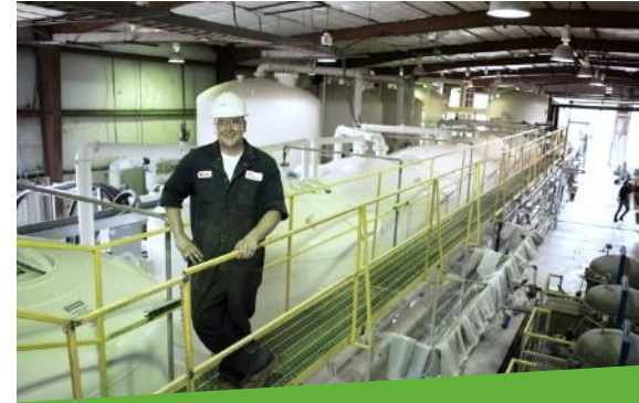
Christensen Satellite Plant
