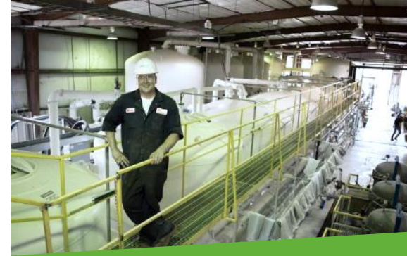
Christensen Satellite Plant
