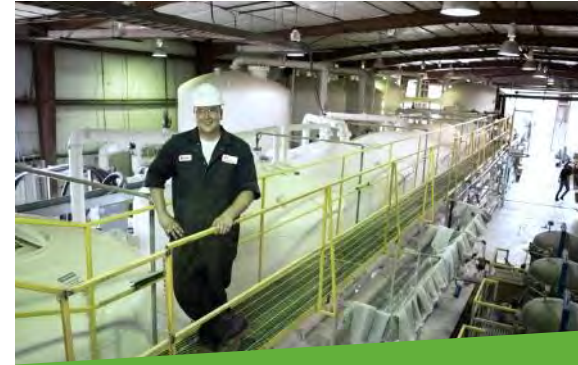
Christensen Satellite Plant
