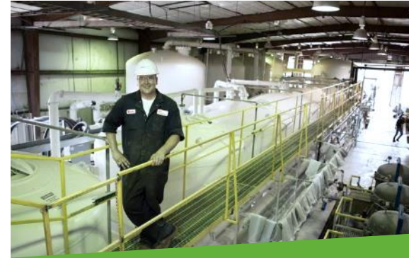
Christensen Satellite Plant
