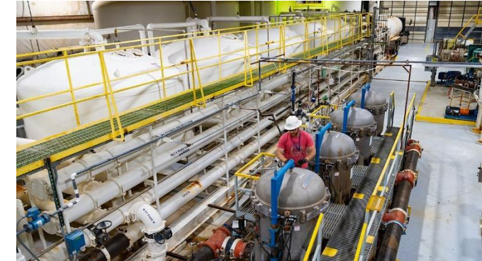
Christensen Satellite Plant Interior
