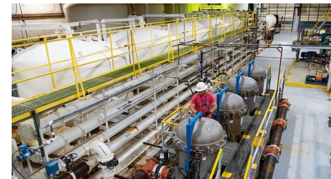
Christensen Satellite Plant Interior
