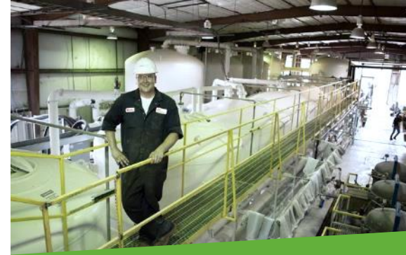
Christensen Satellite Plant
