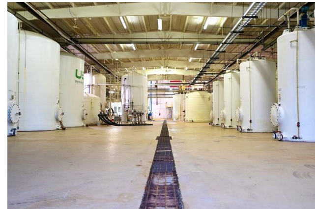
Irigaray CPP Interior, North and South Elution Circuits
