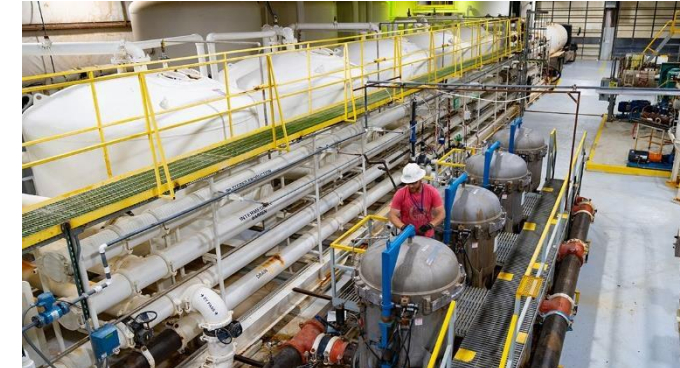
Christensen Satellite Plant Interior
