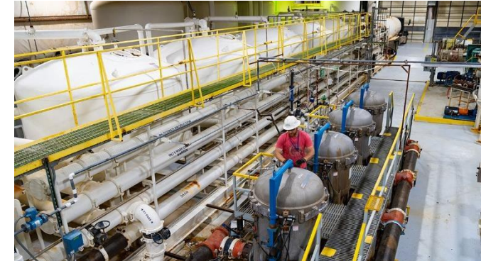
Christensen Satellite Plant Interior
