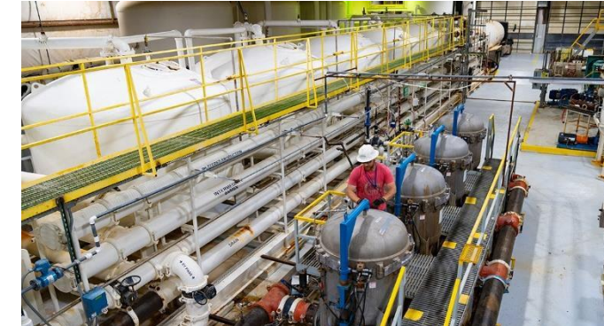
Christensen Satellite Plant Interior
