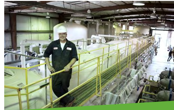
Christensen Satellite Plant
