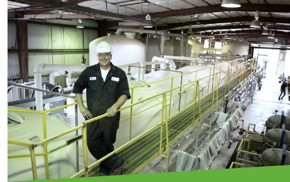
Christensen Satellite Plant
