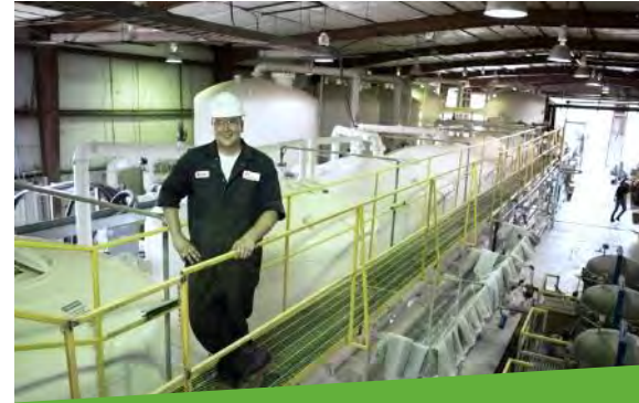
Christensen Satellite Plant
