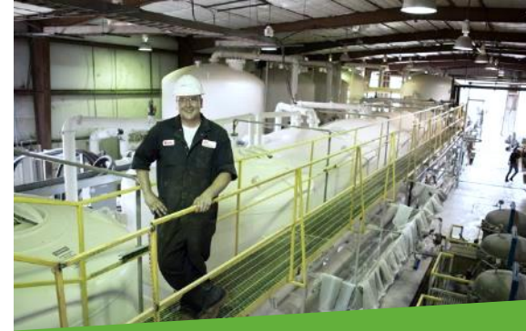
Christensen Satellite Plant
