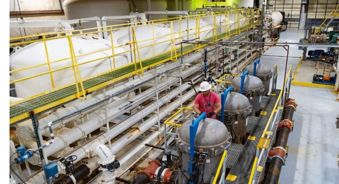
Christensen Satellite Plant Interior
