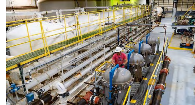
Christensen Satellite Plant Interior
