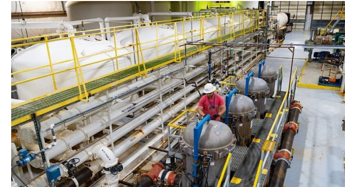
Christensen Satellite Plant Interior
